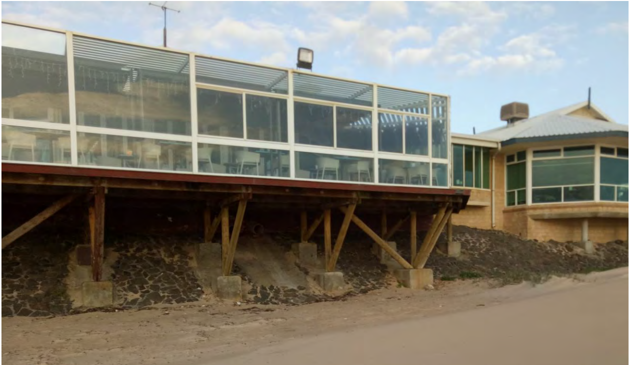
Figure 5-2 Revetment beneath Bunbury Back Beach Café, June 2021.
