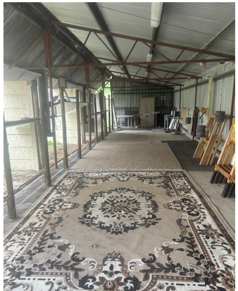
Figure 3 Use of carpets to cover poor floor surface
